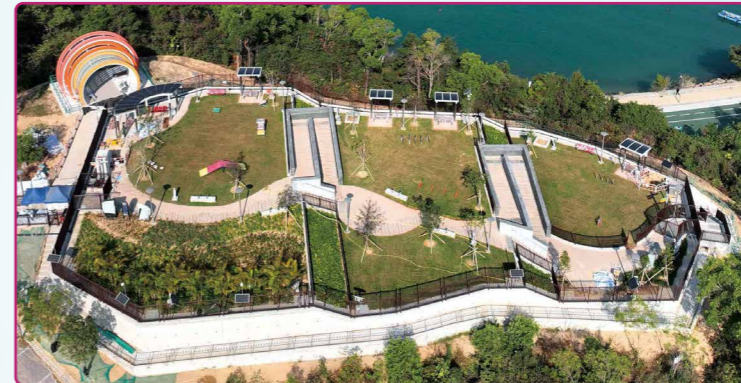
東涌小炮台公園的建造工程已大致完成 The construction work of Tung Chung Battery Park was substantially completed
