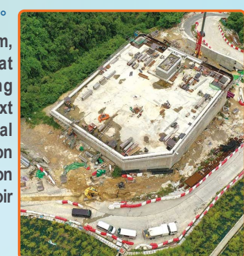
海水配水庫正在建造中 Construction of Salt Water Service Reservoir in progress
