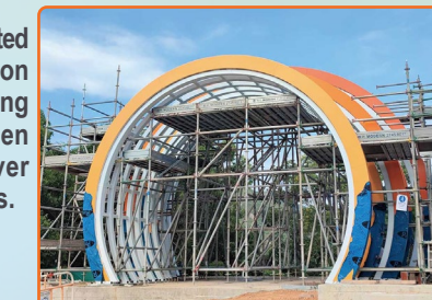
東涌第29A區休憩處正進行涼亭上蓋安裝工程 Roof cover installation for the pavilion at the Open Space of Tung Chung Area 29A
