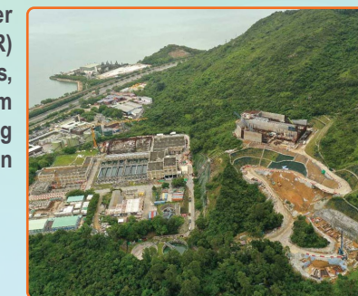
小蠔灣食水配水庫正在建造中 Construction of Siu Ho Wan Fresh Water Service Reservoir in progress
