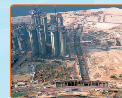
公用設施共同溝現正進行鋼筋混凝土結構工序 The reinforced concrete works at Common Utility Tunnel in progress
