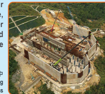
海水抽水站正在建造中 Construction of Salt Water Pumping Station in progress
