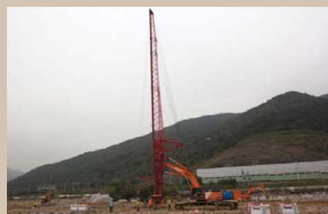
安裝預制垂直排水板將海洋沉積土中的水分排走 Installing prefabricated vertical drains to drain water away from the marine deposit
