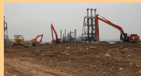
放置公眾填料作為主要的填海物料 Placing public fill as major reclamation material
